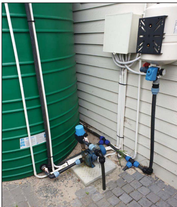
Figure 2-5 A private groundwater use at a household where a borehole is used for non-potable, domestic supply. The borehole headworks, with a large JoJo tank for storage, as well as a small filter and treatment system are noted.
